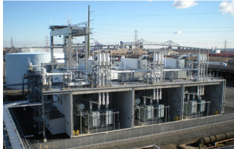
One of Linden VFT's variable-frequency transformers in Linden, N.J. | Joseph Jingoli & Son
